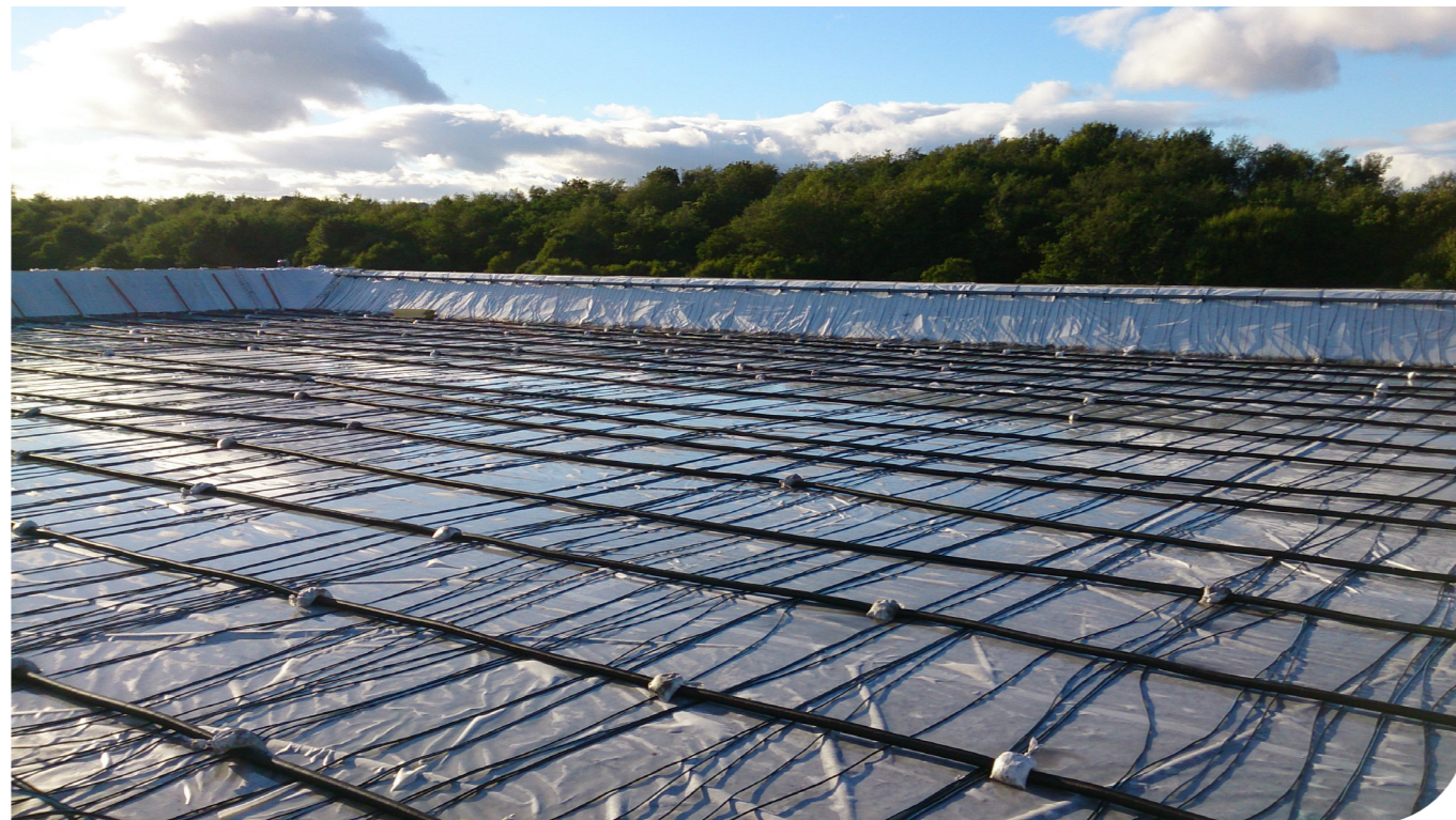
Collection pipework and airline installation
